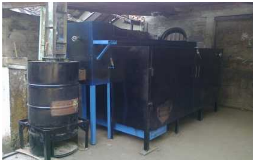
Figure 4. Development of wood drying kiln.
